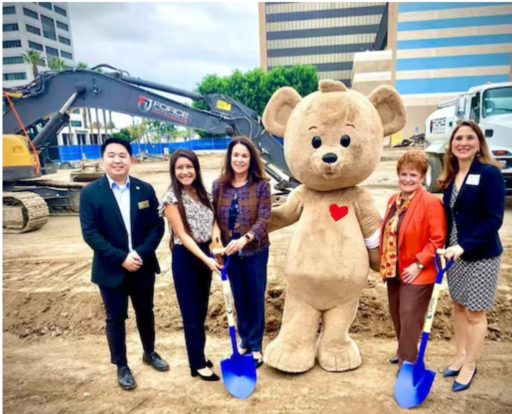
Team Wagner Field Representative Pat Buttress helps break ground for the new CHOC Children's Hospital Southwest Tower. It will open in phases and include a Research Institute with outpatient infusion therapies, radiology, and beyond. We are grateful to have this community resource in our backyard in the City of Orange. Follow the journey #longlivechildhood.
